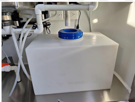
- Clean Water Tank -
